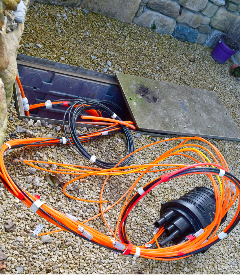
Access and joining box in the ground
